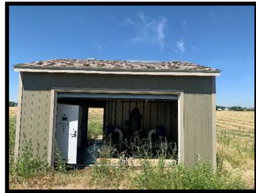
West Milavec Pump Station
