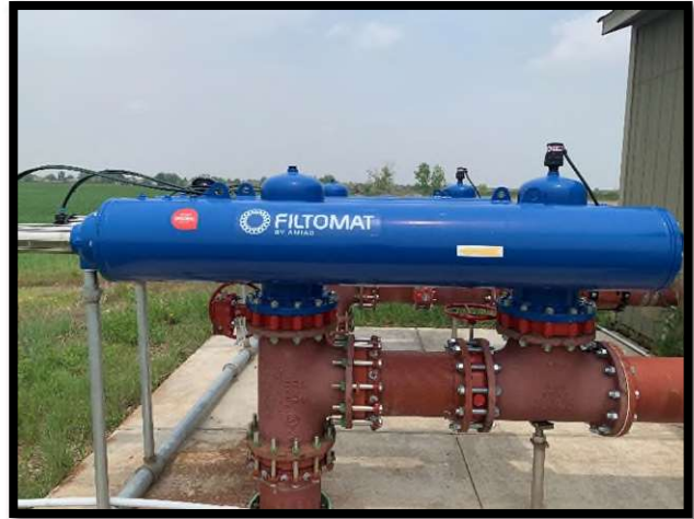
West Milavec Pump Station Filters
